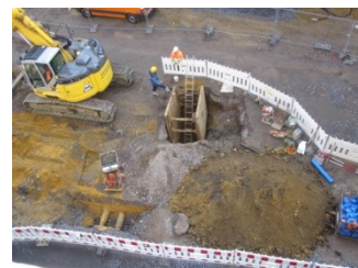
It did not take long before the trench protection could be installed ..
